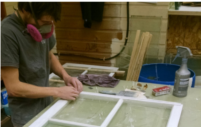
Many wood windows can be rehabilitated by repairing wood sashes, replacing glazing, and installing new putty.
