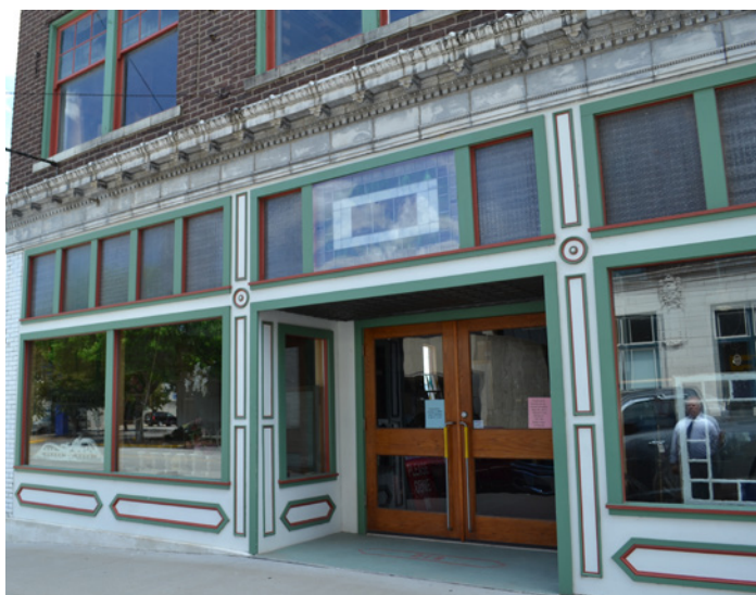
This reconstructed wood storefront contains traditional elements, highlighted by a three-tone color scheme. Page 126
