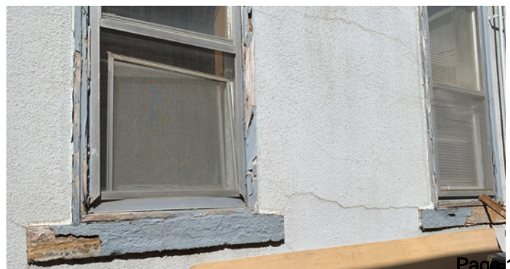
Deferred window maintenance is unsightly and can also affect the thermal performance of a building.
