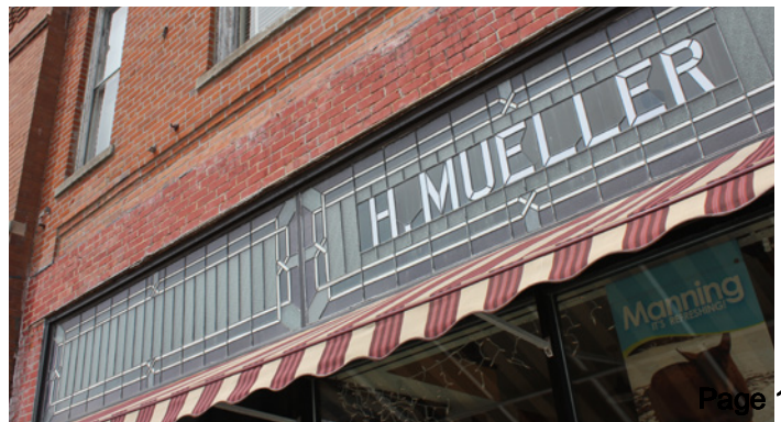
Historic transoms are sometimes highly decorative and can contain historic business signage or building names.
