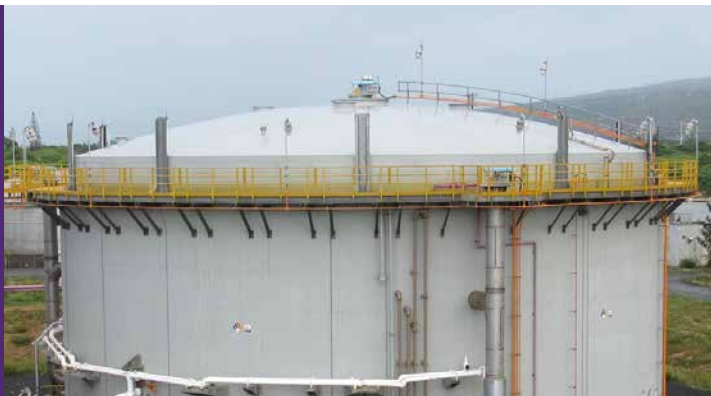
Honouliuli WWTP, HI (90' G2VL): Gasholder Steel Cover
